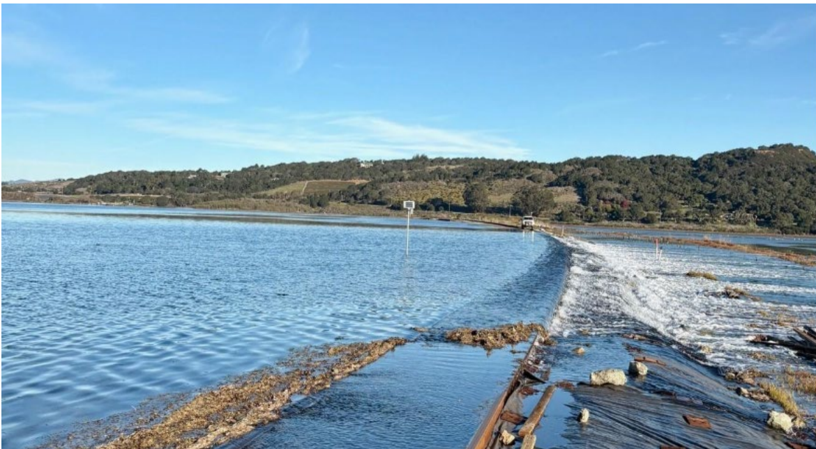
View of overtopped active rail corridor at Elkhorn Slough.
